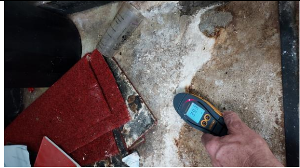
High moisture reading to some floors.
